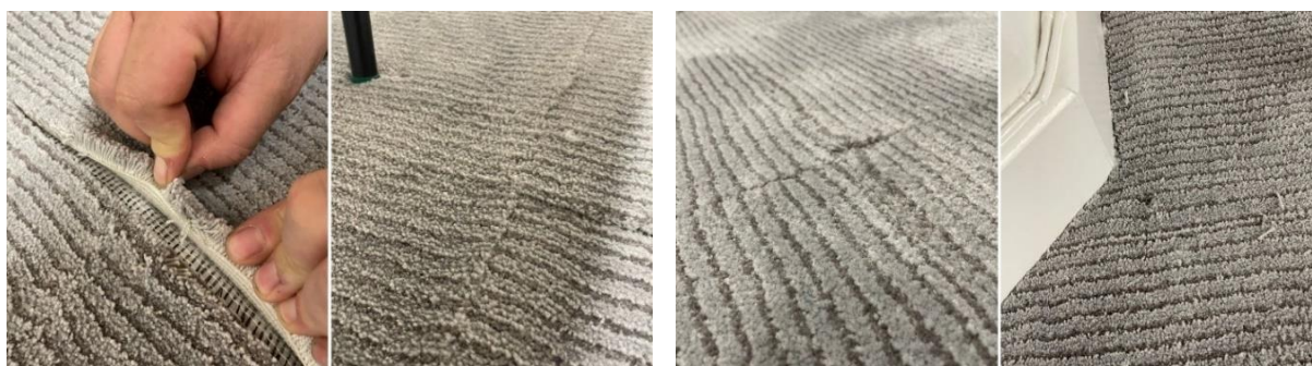
Figure 19: Stage 2 cTextile installation issues
